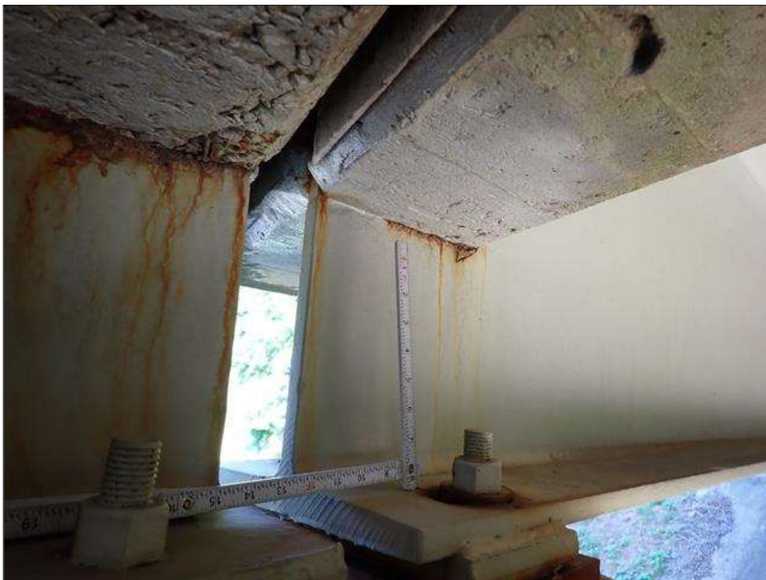
Span 4 Beam 1: at bent 3, corrosion with section loss: web adjacent to end diaphragm (9/16 inch average remaining x 10 inch x 1 inch)
