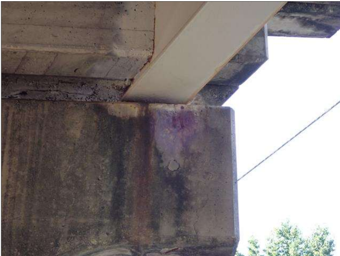
Bent 3 Cap 1: NORTH FACE OF CAP UNDER BEAM 1 HAS A 9 INCH X 11 INCH X 2 INCH DEEP SPALL AT TOP OF CAP.
