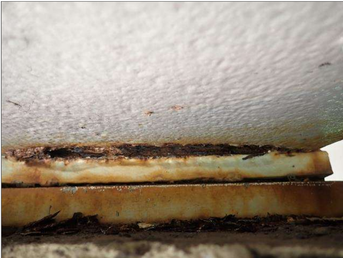
Span 3 Beam 2: at bent 2, corrosion with section loss: web adjacent to end diaphragm (9/16 inch average remaining x 10 inch x 4 inch); bottom flange (0.80 inch average remaining x 1 inch)
