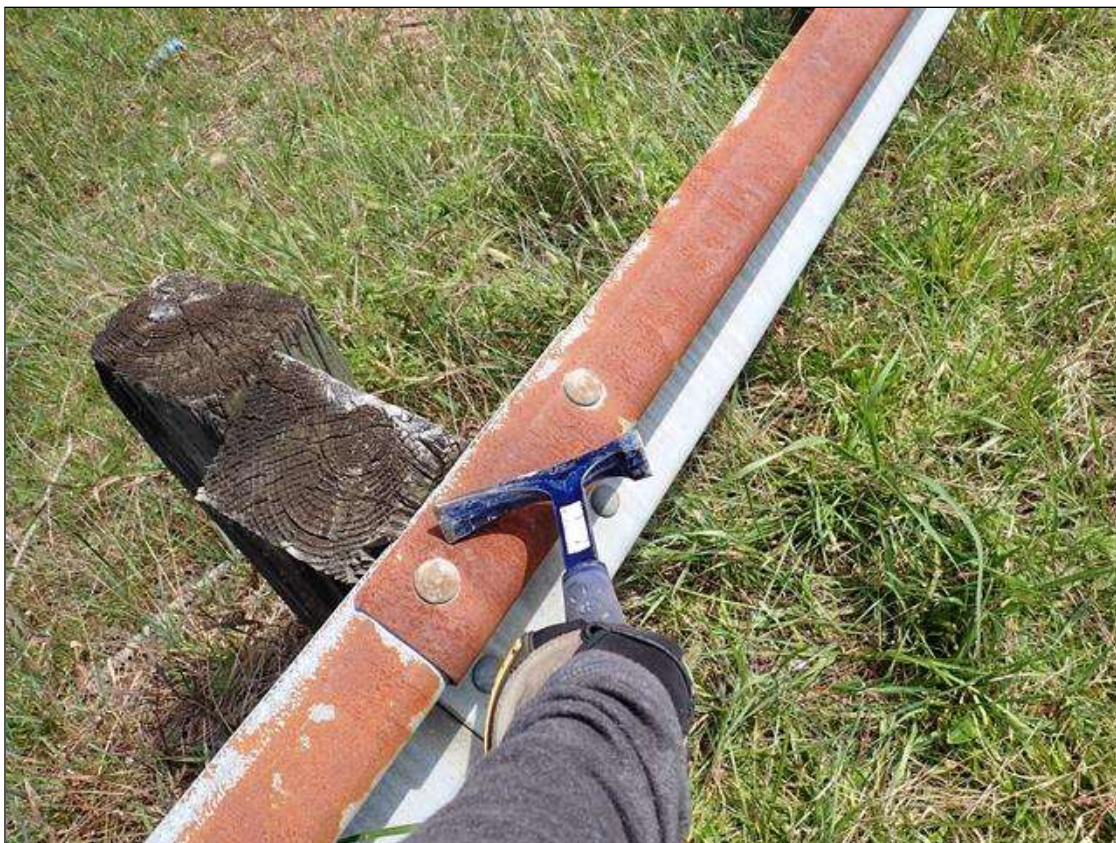
along all guardrails, surface rust at random
