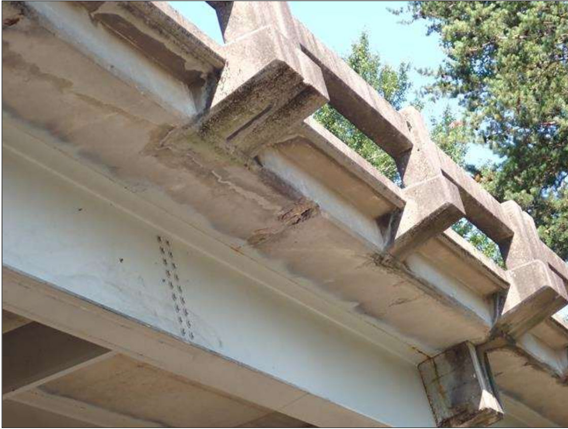
Span 3 Deck: (PAR) MULTIPLE UP TO 1 FOOT X 1 FOOT X 1 INCH DEEP SPALLS/DELAMINATIONS WITH EXPOSED REBAR AT RANDOM THROUGHOUT EAST OVERHANG; SOME DELAMINATIONS OVER TRAVEL LANE
