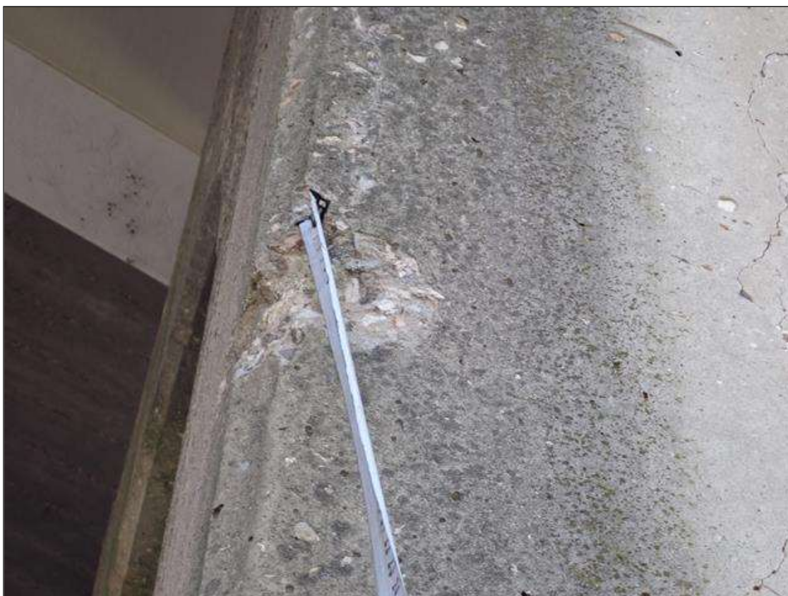
Bent 1 Pile 1: 6 INCH X 6 INCH X 1 INCH DEEP CORNER SPALL NORTHWEST CORNER 5 foot FROM BOTTOM OF CAP
