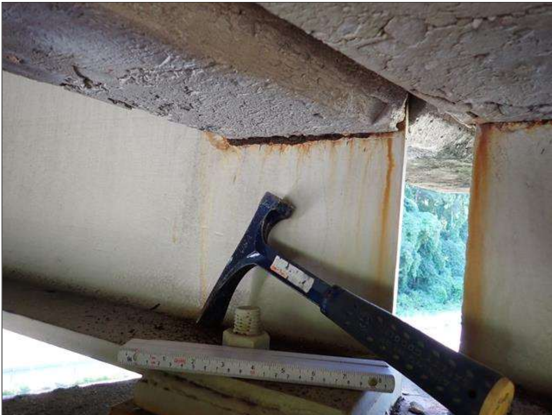
Span 2 Beam 1: at bent 2, corrosion with section loss: web adjacent to end diaphragm (9/16 inch average remaining x 10 inch x 3 inch)
