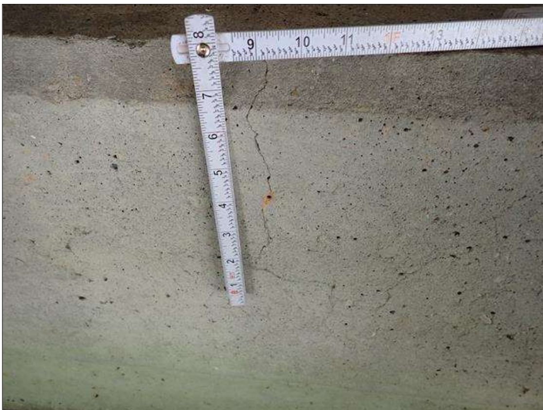
End Bent 1 Cap 1: along length, multiple vertical cracks [up to full height x 1/32 inch]
