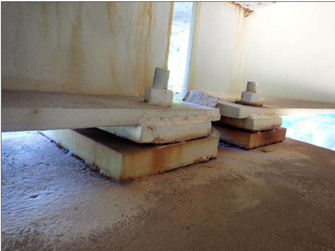
interior bearing assembly
