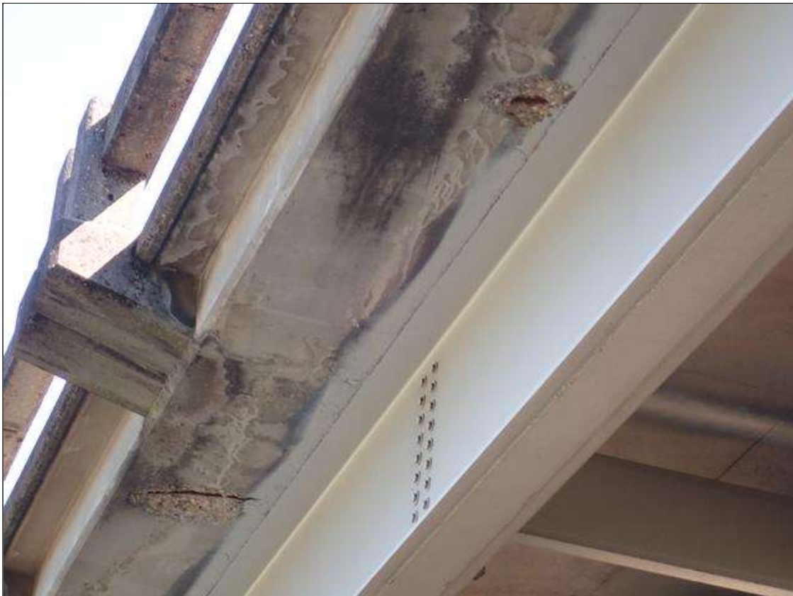
Span 3 Deck: (PAR) MULTIPLE UP TO 2 FOOT X 1 FOOT X 1 DEEP SPALL/DELAMINATION WITH EXPOSED REBAR AT RANDOM THROUGHOUT WEST OVERHANG; SOME DELAMINATION OVER TRAVEL LANES
