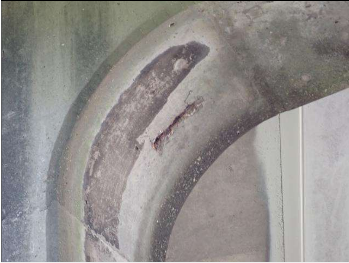
Bent 1 Cap 1: BOTTOM FACE OF CAP RIGHT SIDE OF COLUMN 1 HAS A SURFACE SPALL AREA 3 INCH WIDE X 10 INCH LONG X 1/2 INCH DEEP WITH REBAR EXPOSED.
