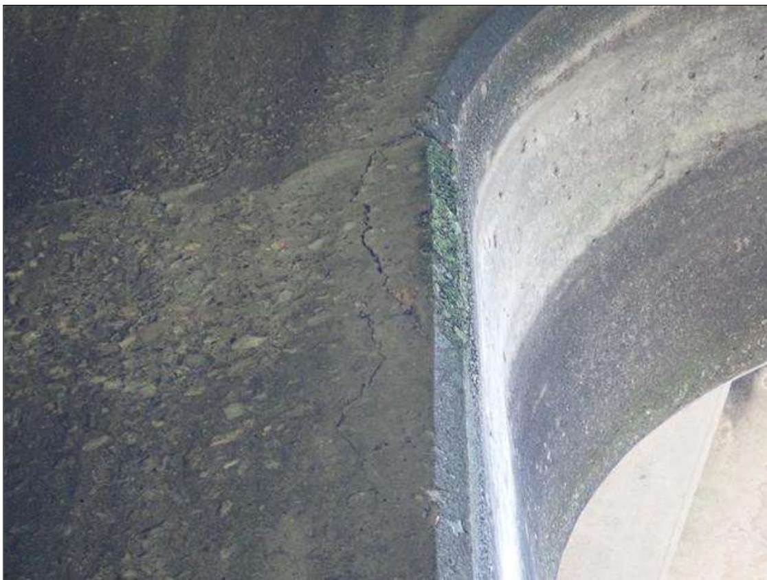
Bent 1 Pile 2: UP TO 3 FOOT X 1/16 INCH VERTICAL CRACKS ALL FACES NEAR BOTTOM OF CAP
