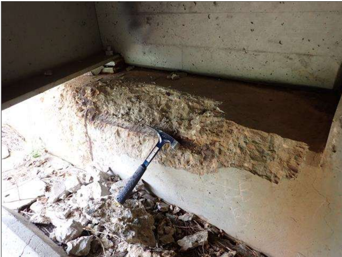
End Bent 2 Cap 1: (PAR) 6 FOOT X UP TO 16 INCH X 10 INCH X 3 INCH DEEP SPALL WITH EXPOSED PRIMARY REBAR WITH SECTION LOSS [UP TO 1/16 INCH] UNDER BEAM 1
