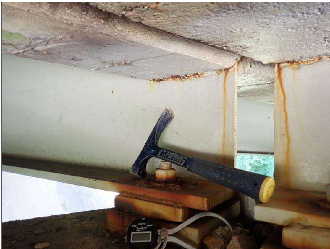
Span 1 Beam 3: at bent 1, corrosion with section loss: web adjacent to end diaphragm (9/16 inch average remaining x 10 inch x 1 inch)
