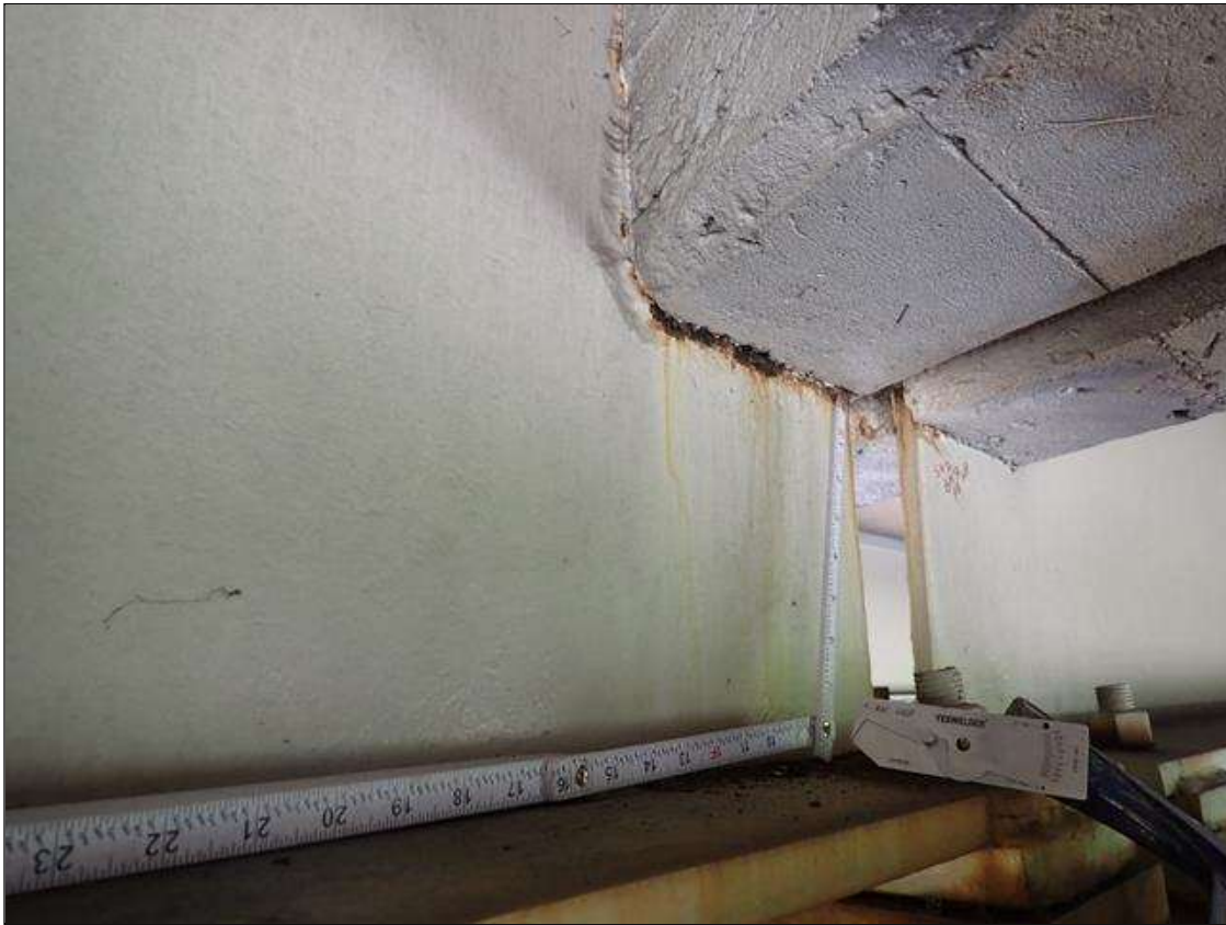
Span 3 Beam 2: at bent 2, corrosion with section loss: web adjacent to end diaphragm (9/16 inch average remaining x 10 inch x 4 inch); bottom flange (0.80 inch average remaining x 1 inch)
