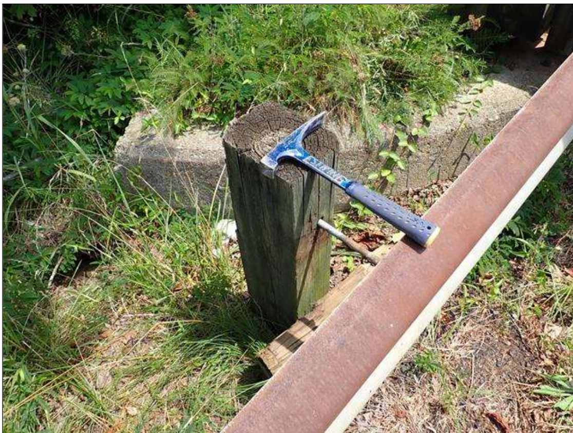
(PAR) northeast guardrail, 3rd and 7th timber posts from end bent 2, timber spacers, missing
