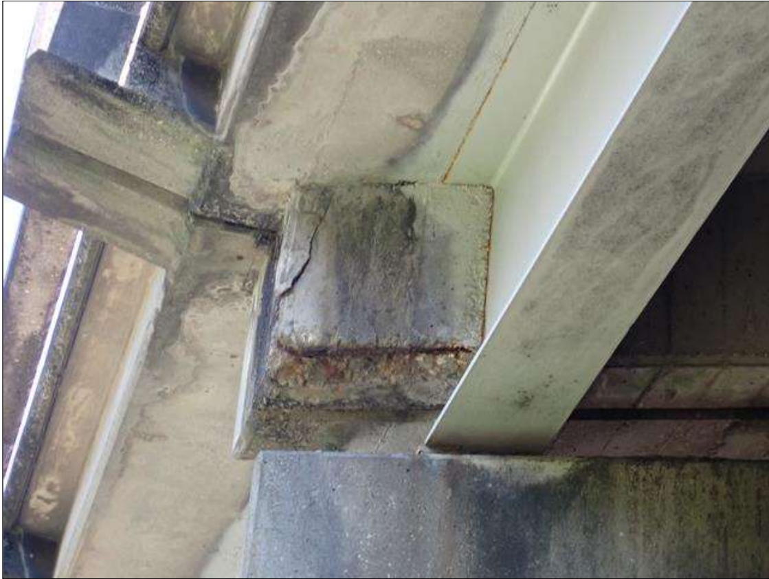
Span 1 Beam 1: (PAR) 2 FOOT X UP TO 1 FOOT X 2 INCH DEEP DIAPHRAGM SPALL/DELAMINATION WITH EXPOSED REBAR WITH APPROXIMATELY 25 PERCENT LOSS WEST OVERHANG AT BENT 1.
