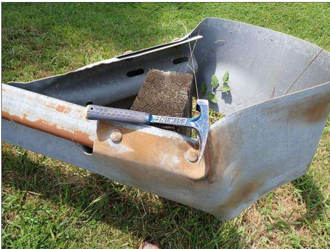
(PAR) northwest guardrail termination, impact damage
