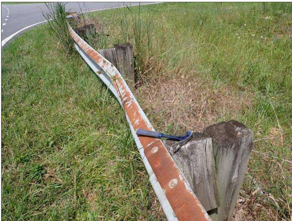
(PAR) northeast guardrail 18 foot from termination, impact damage (7 foot)
