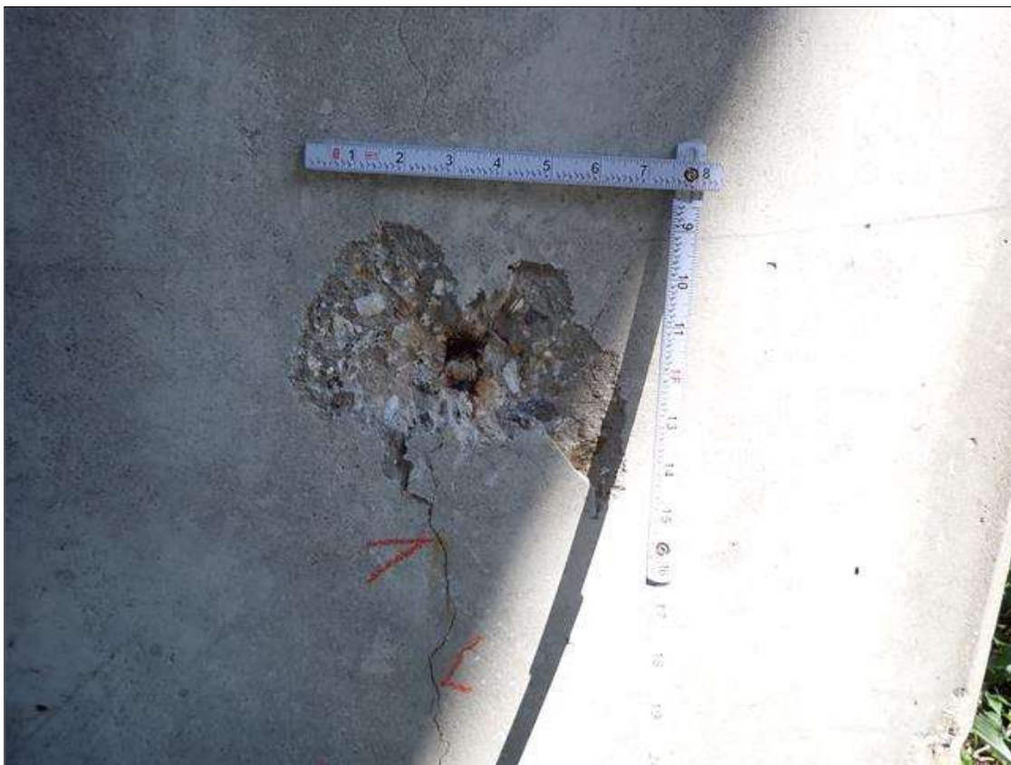
Bent 2 Pile 2: South face starting at ground line, vertical crack (1/32 inch x full height); 2 foot from ground, spall (8 inch x 5 inch x 1/2 inch deep) with exposed rusted rebar
