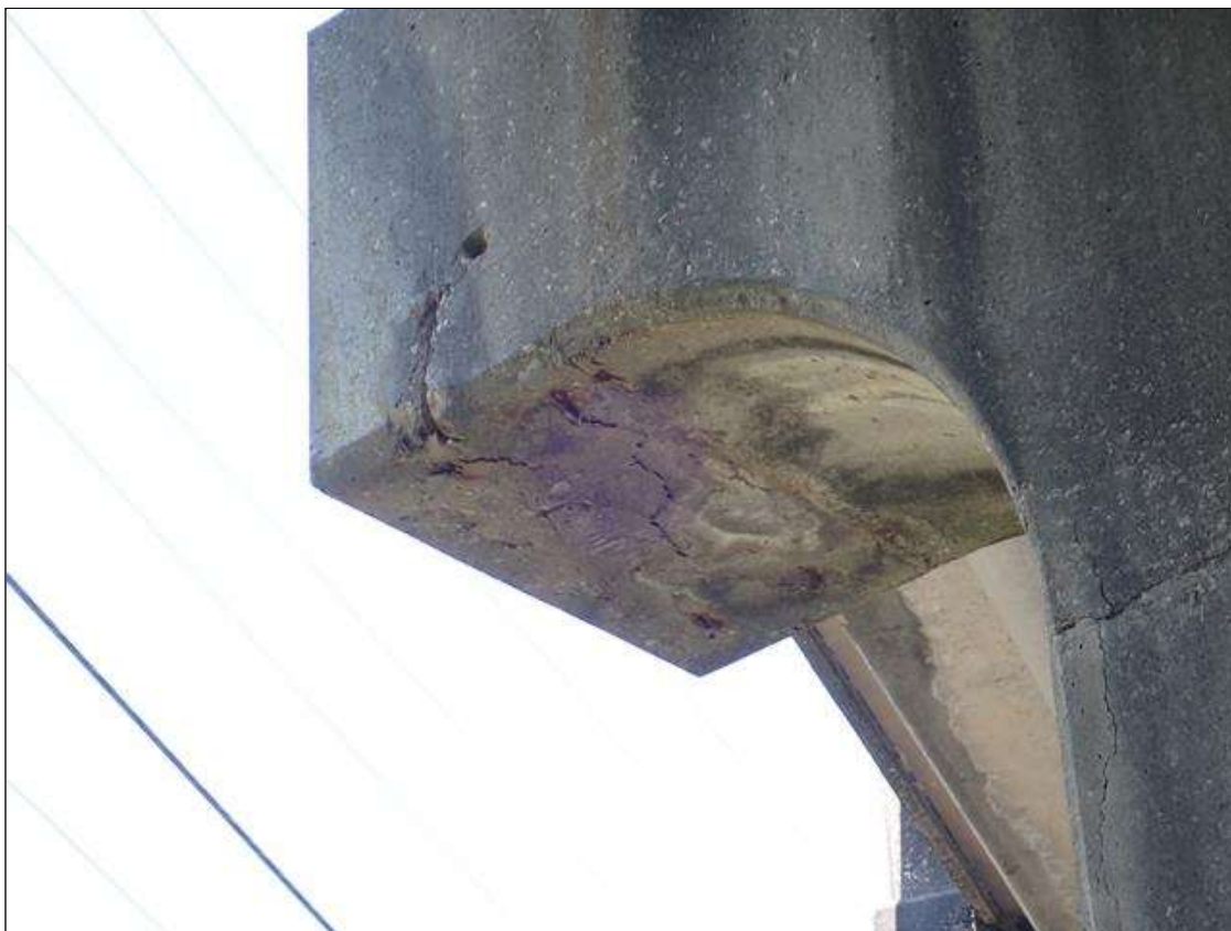
Bent 1 Cap 1: South face at West end, spall [15 inch x 3 inch x 1 inch deep] with exposed rusted reinforcing [no loss] and adjacent delamination at underside [1 foot x full width]
