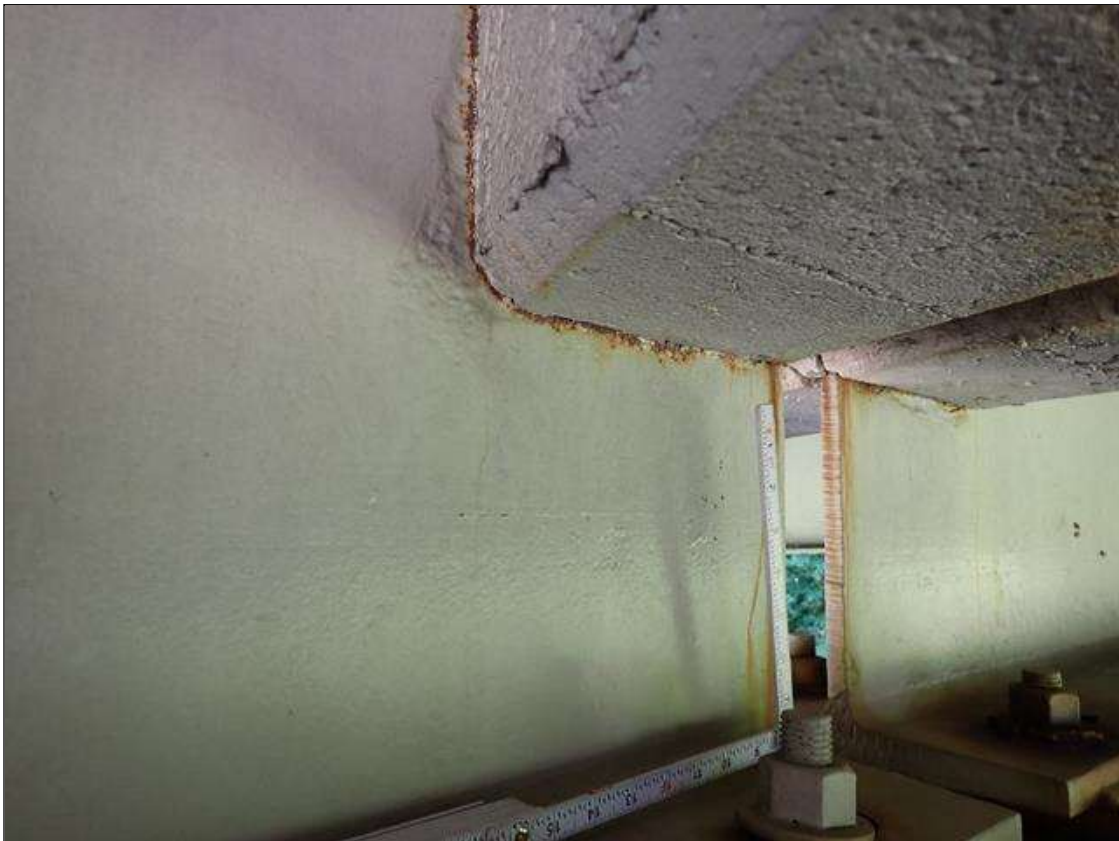
Span 2 Beam 2: at bent 1, corrosion with section loss: web adjacent to end diaphragm (9/16 inch average remaining x 10 inch x 4 inch)
