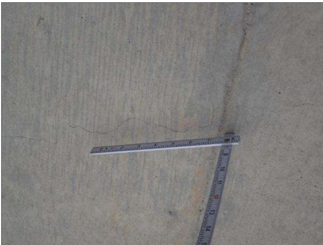
Span 1 Deck: throughout underside of all bays, multiple transverse cracks [up to 8 foot x 1/32 inch] and map cracks (hairline) at random
