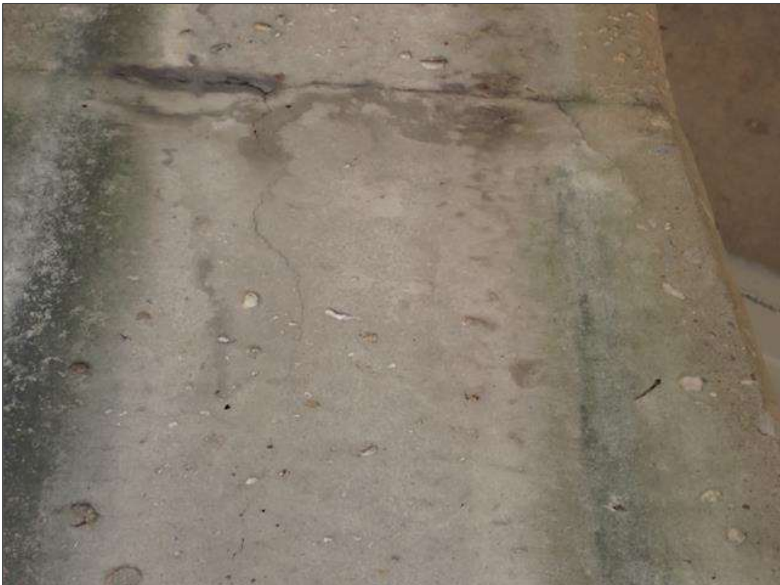
Bent 3 Pile 1: at West face, (2) vertical cracks [up to 3 foot x 1/32 inch]
