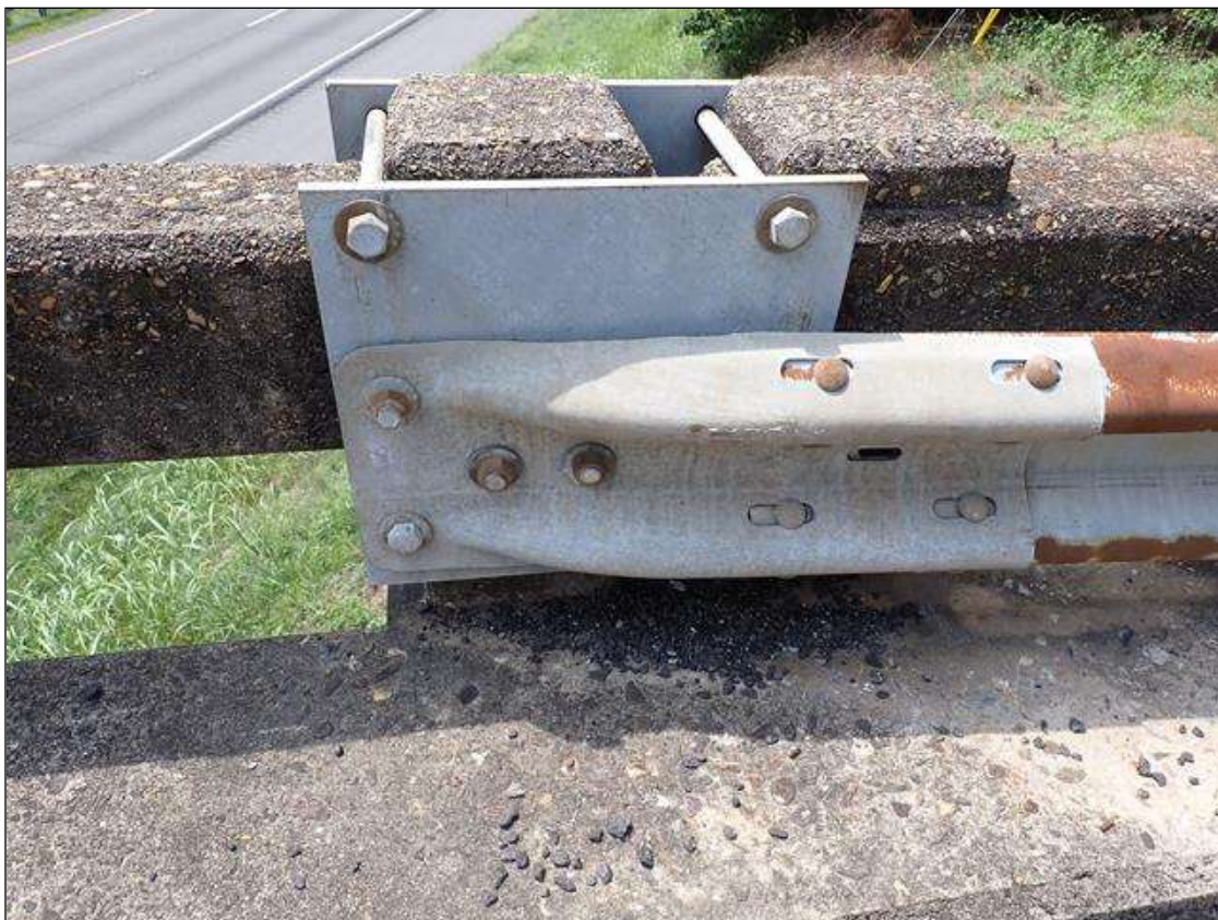
(PAR) northwest guardrail attachment, improper lap
