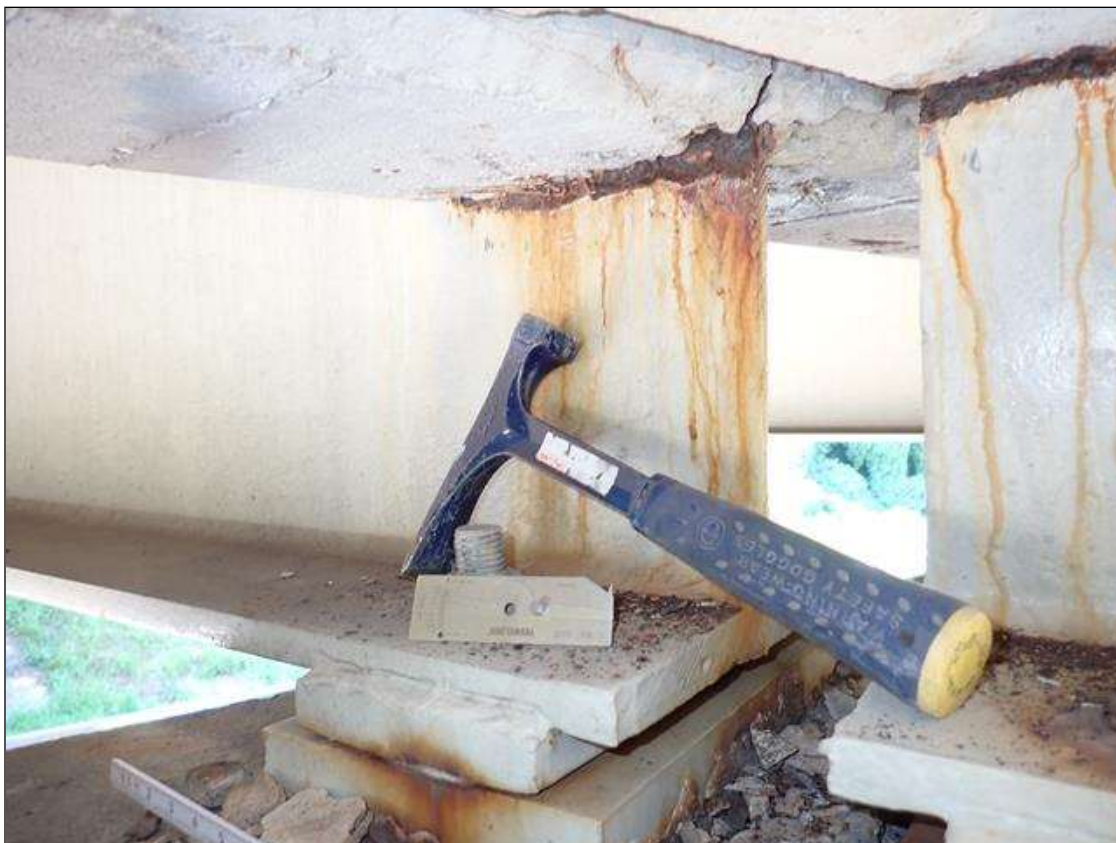
Span 2 Beam 3: at bent 2, active corrosion with section loss, web at diaphragm [9 inch x 1 inch x average remaining 1/2 inch]
