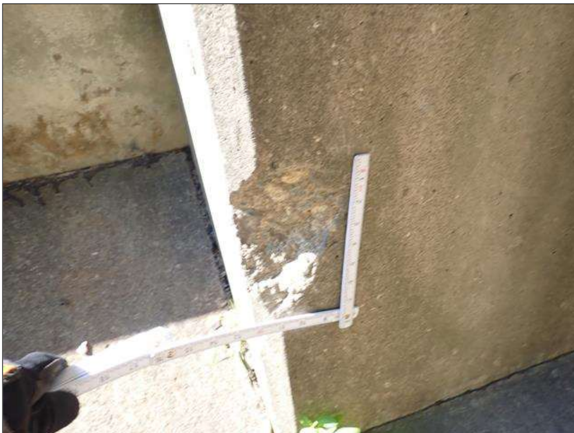
Bent 3 Pile 2: BOTTOM OF COLUMN 2 NORTHEAST CORNER HAS A SPALL AREA 5 INCH X 8 INCH X 1 INCH DEEP.
