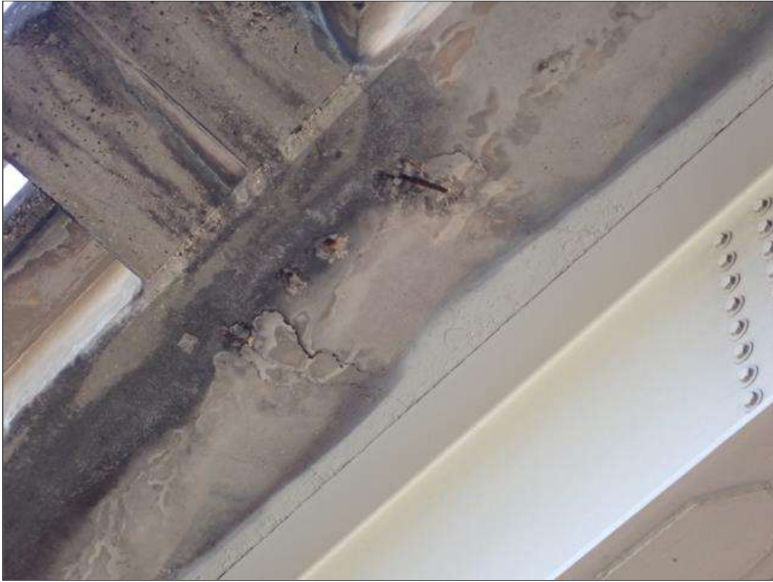
Span 3 Deck: (PAR) MULTIPLE UP TO 2 FOOT X 1 FOOT X 1 DEEP SPALL/DELAMINATION WITH EXPOSED REBAR AT RANDOM THROUGHOUT WEST OVERHANG; SOME DELAMINATION OVER TRAVEL LANES
