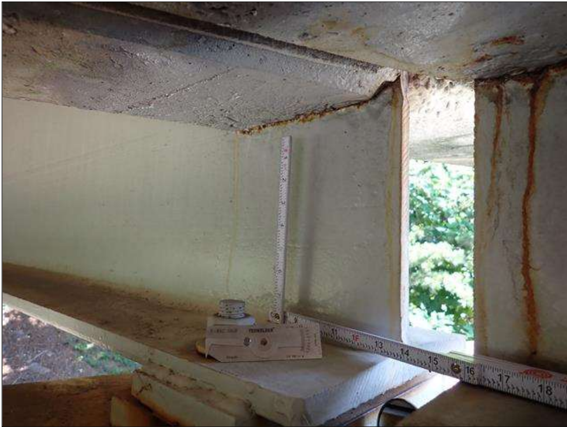
Span 4 Beam 4: at bent 3, corrosion with section loss: web adjacent to end diaphragm (9/16 inch average remaining x 10 inch x 1 inch)
