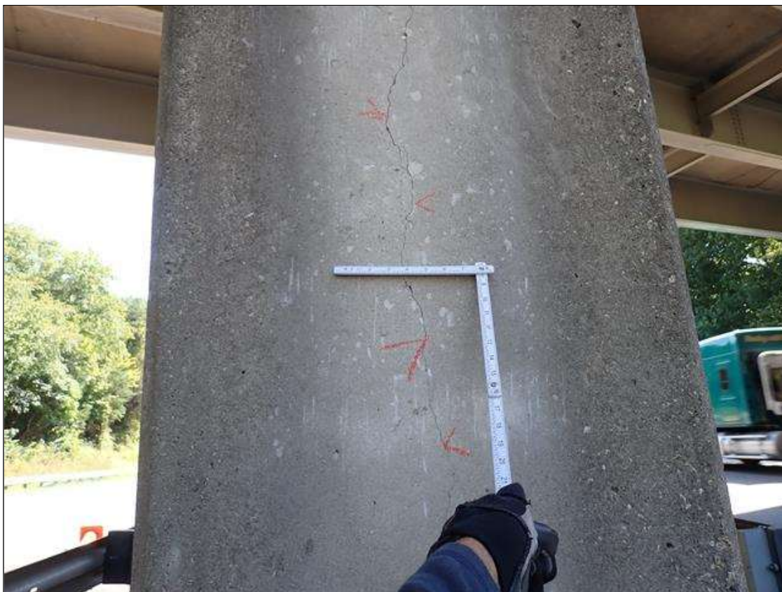
Bent 2 Pile 1: FULL HEIGHT X UP TO 1/32 INCH VERTICAL CRACKS WEST AND NORTH FACES BEGINNING AT BOTTOM OF CAP
