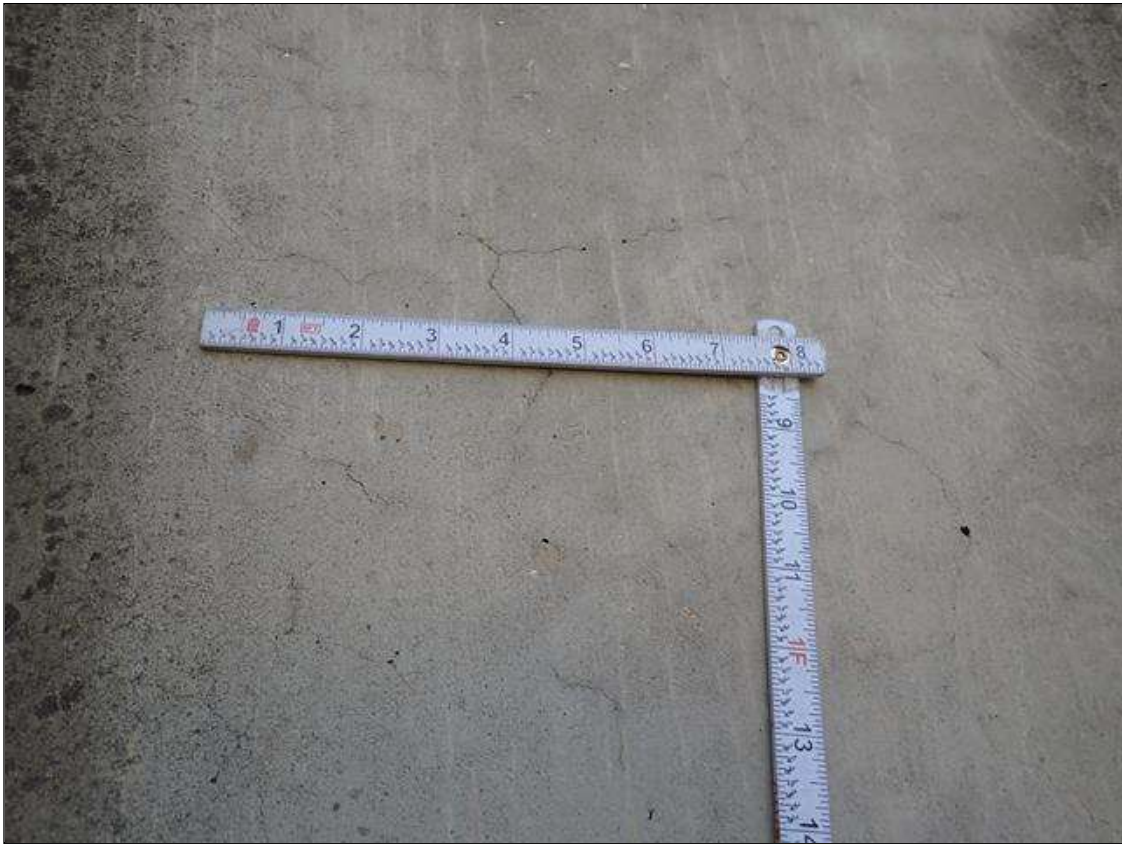
Bent 3 Pile 1: at East face, hairline map cracking at random
