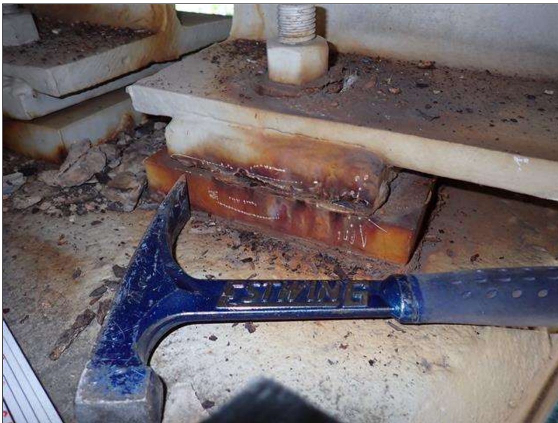
Span 3 Beam 3 - Near Bearing 3: rust scale
