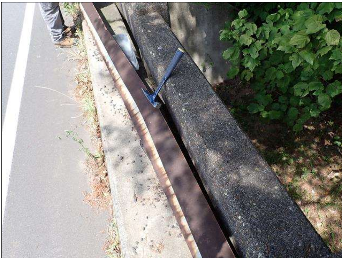
(PAR) northeast guardrail 4 foot from attachment, impact damage (6 foot)
