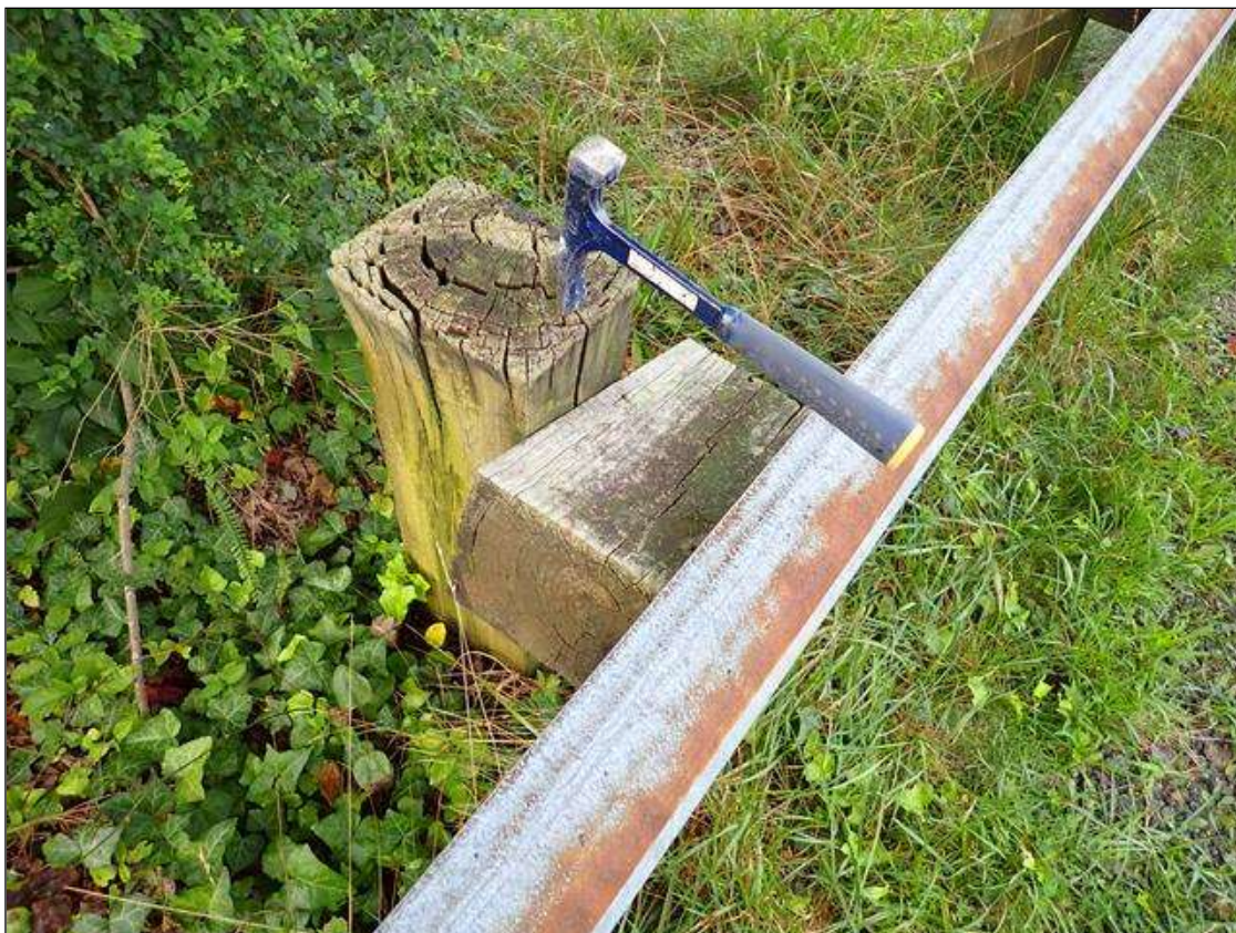
(PAR) along all guardrails, timber spacers, loose/twisted
