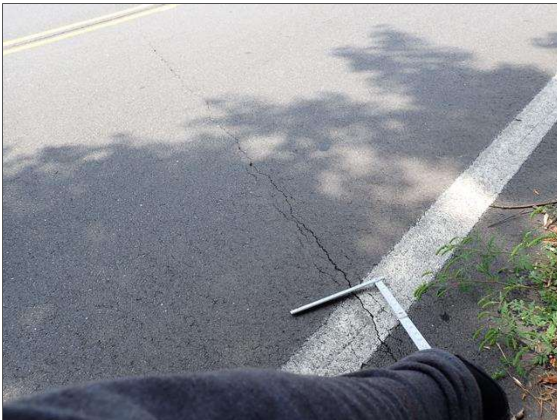
Span 1 Wearing Surface: over end bent 1, right travel lane, transverse crack (1/16 inch x 12 foot)
