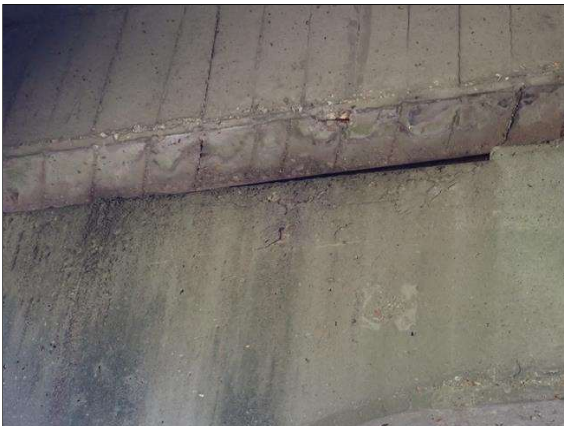
Bent 1 Cap 1: BENT 1 SOUTH FACE OF CAP BETWEEN BEAM 1 AND BEAM 2 CRACKED AND DELAMINATED AREA TOP FACE OF CAP 11 INCH X 31 INCH
