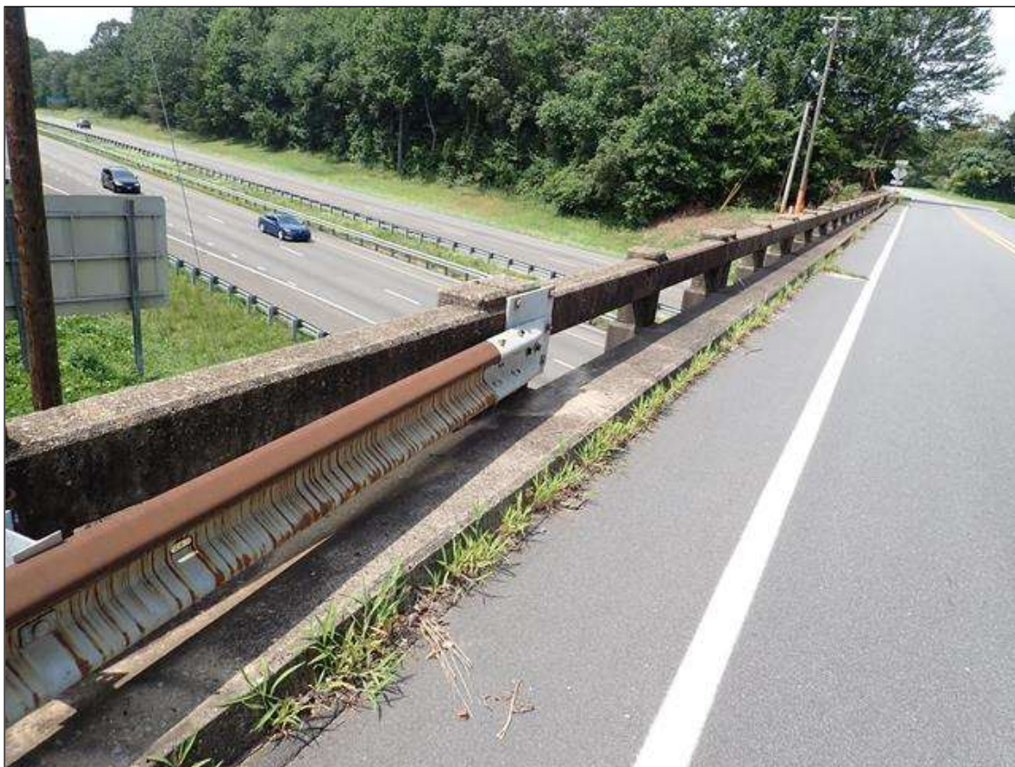
left bridge rail
