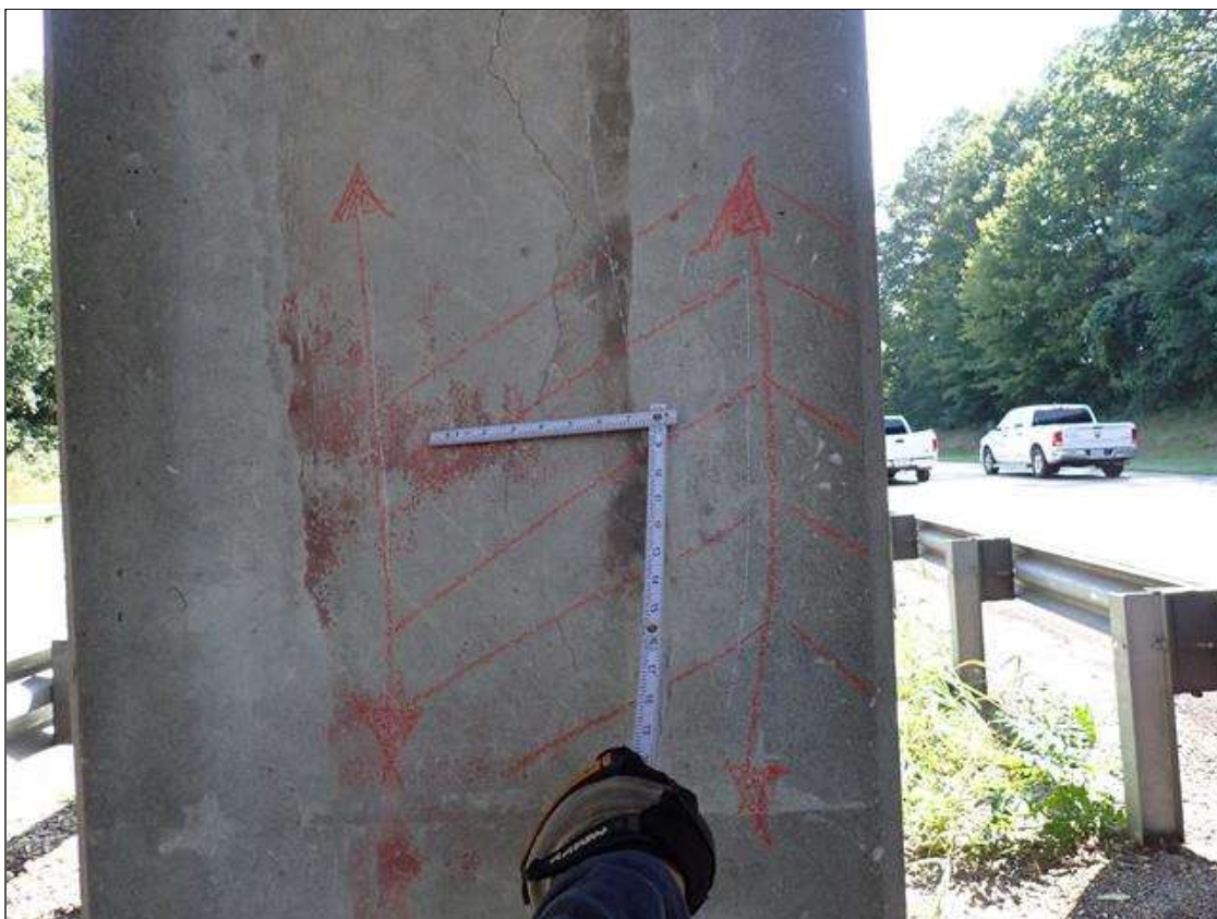
Bent 2 Pile 2: West face mid height, delamination [6 foot x 18 inch] with cracks [up to 1/32 inch]
