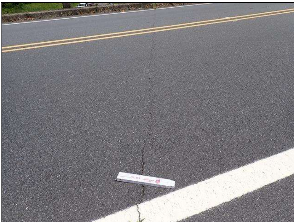
Span 2 Wearing Surface: over bent 1, transverse crack (up to 1/16 inch x 28 foot)
