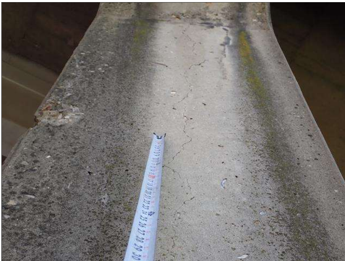
Bent 1 Pile 1: UP TO 7 FOOT X UP TO 1/16 INCH VERTICAL CRACKS WEST AND EAST FACES
