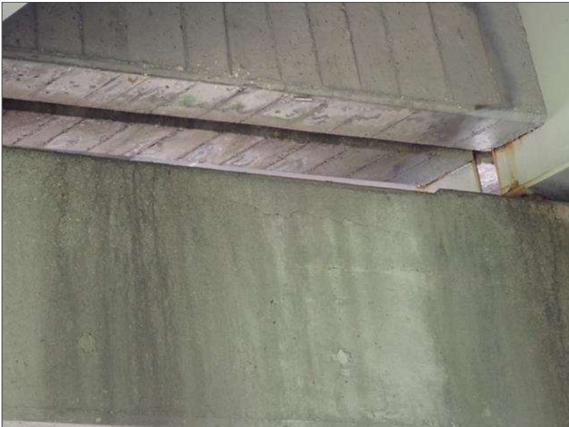
Bent 1 Cap 1: BENT 1 SOUTH FACE OF CAP HAS A HORIZONTAL CRACK UP TO 1/32 INCH X 3 FOOT ALONG TOP EDGE BETWEEN BEAMS 2 AND BEAMS 3.
