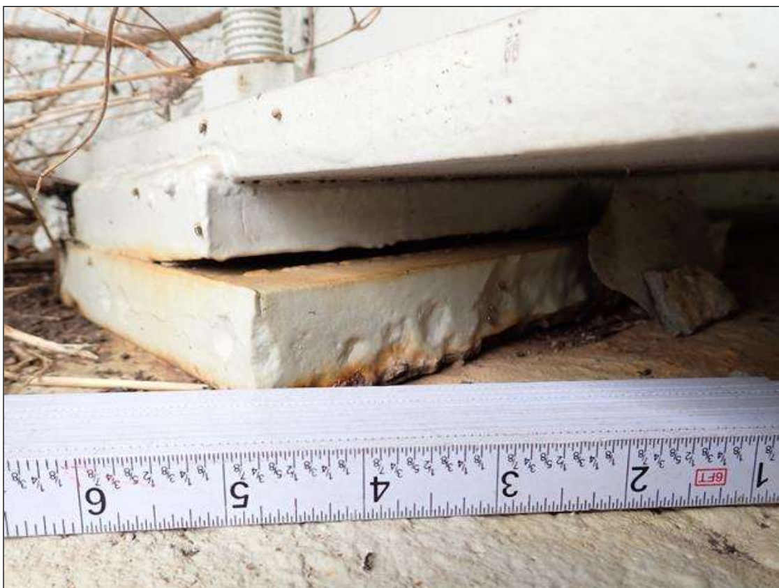
Span 4 Beam 1 - Far Bearing 1: painted over section loss (up to 1/8 inch deep) with corrosion reactivating
