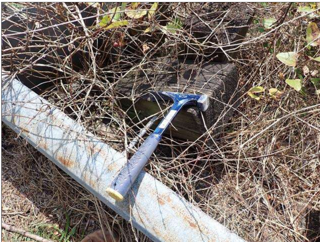
(PAR) northwest guardrail, 1st, 7th and 8th timber posts from end bent 2, timber spacers, missing
