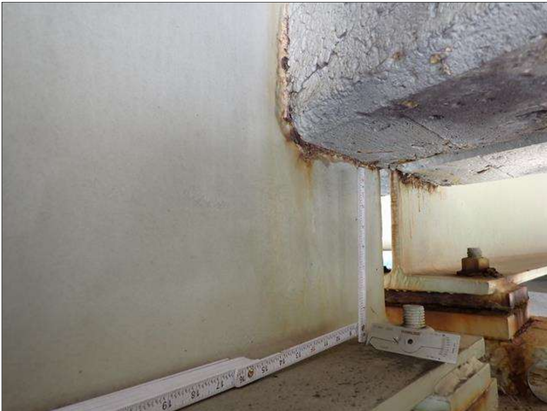
Span 3 Beam 3: at bent 3, corrosion with section loss: web adjacent to end diaphragm (1/2 inch average remaining x 10 inch x 6 inch)
