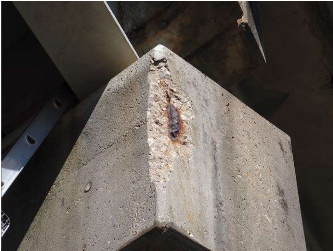
Bent 3 Cap 1: (PAR) 12 INCH X 24 INCH X 2 INCH DEEP SPALL WITH EXPOSED REBAR WITH APPROXIMATELY 25 PERCENT LOSS SOUTHEAST CORNER
