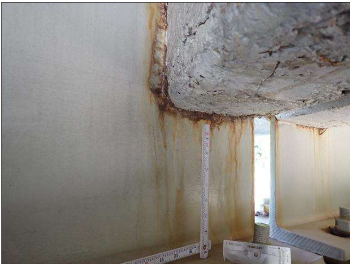
Span 3 Beam 1: at bent 3, corrosion with section loss: web adjacent to end diaphragm (1/2 inch average remaining x 10 inch x 9 inch)
