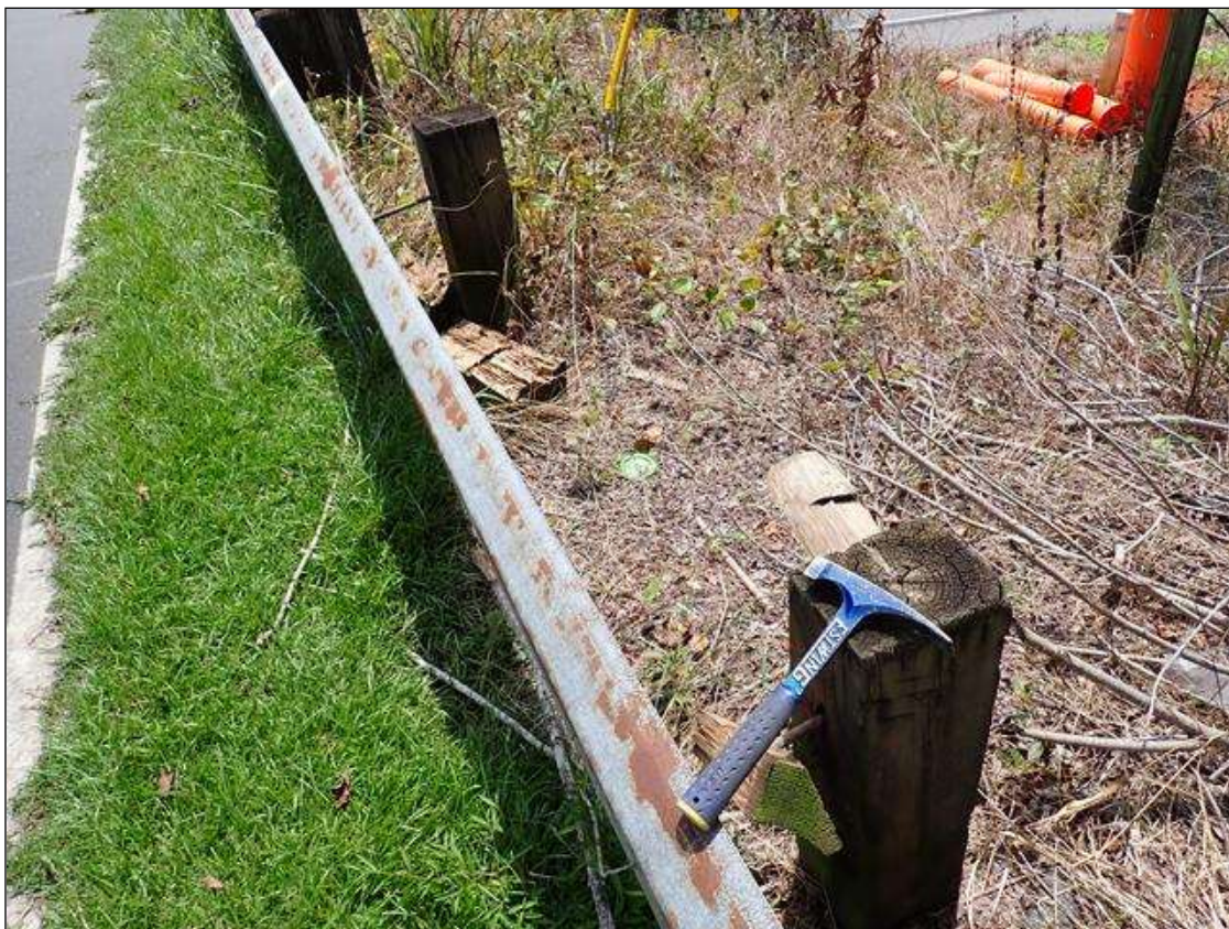
(PAR) northwest guardrail, 1st, 7th and 8th timber posts from end bent 2, timber spacers, missing
