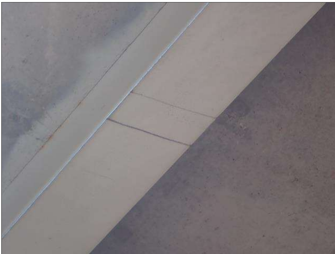
Span 3 Beam 4 - Protective System: over right travel lane, impact scrapes
