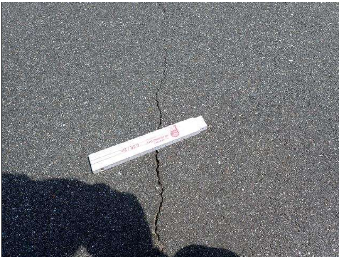
Span 3 Wearing Surface: over bent 2, transverse crack (1/16 inch x 28 foot)
