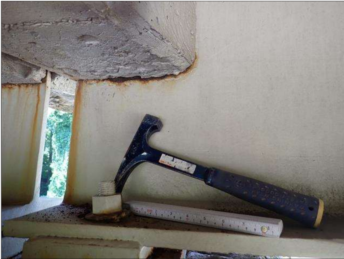
Span 3 Beam 1: at bent 2, corrosion with section loss: web adjacent to end diaphragm (9/16 inch average remaining x 10 inch x 3 inch)
