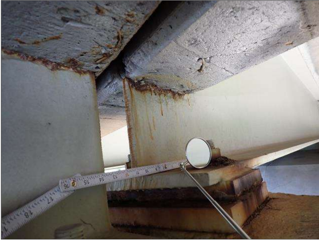
Span 4 Beam 3: at bent 3, corrosion with section loss: web adjacent to end diaphragm (1/2 inch average remaining x 10 inch x 1 inch)
