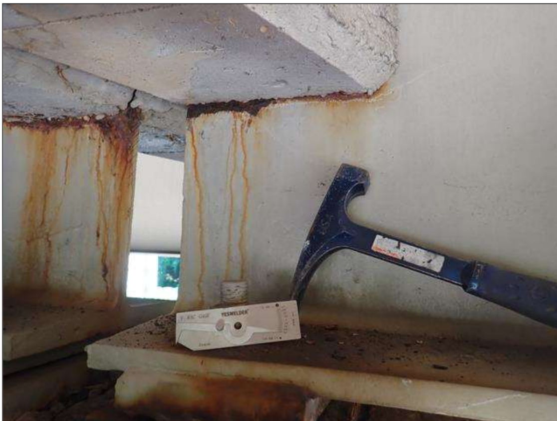
Span 3 Beam 3: at bent 2, active corrosion with section loss, web at diaphragm [10 inch x 1 inch x average remaining 9/16 inch]
