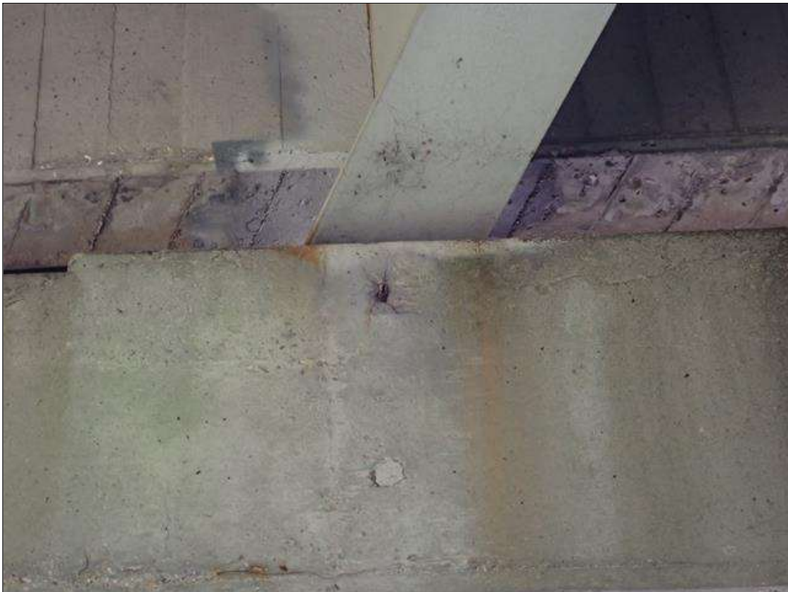
Bent 1 Cap 1: 6 INCH DIAMETER X 1/2 INCH DEEP SPALL WITH EXPOSED REINFORCING SOUTH FACE OF CAP BELOW BEAM 2
