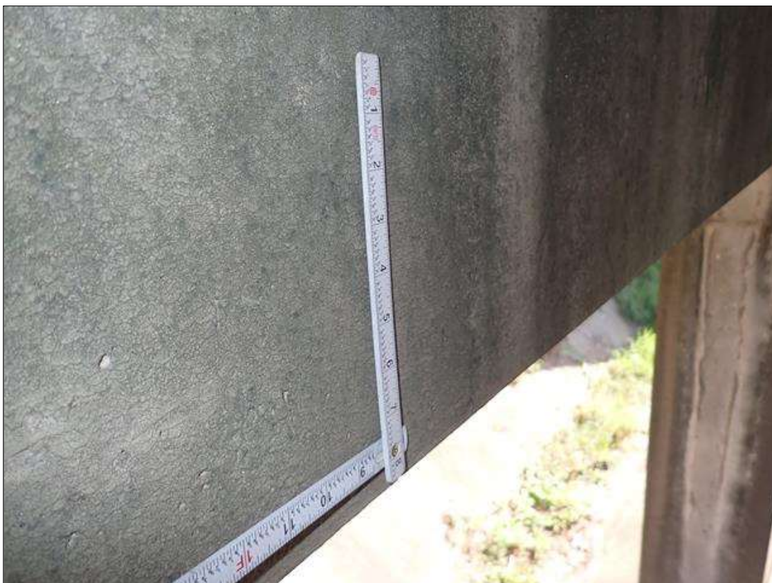
Bent 3 Cap 1: along the length of the cap, vertical cracks (up to 1/32 inch x full height) and map cracks (hairline) at random
