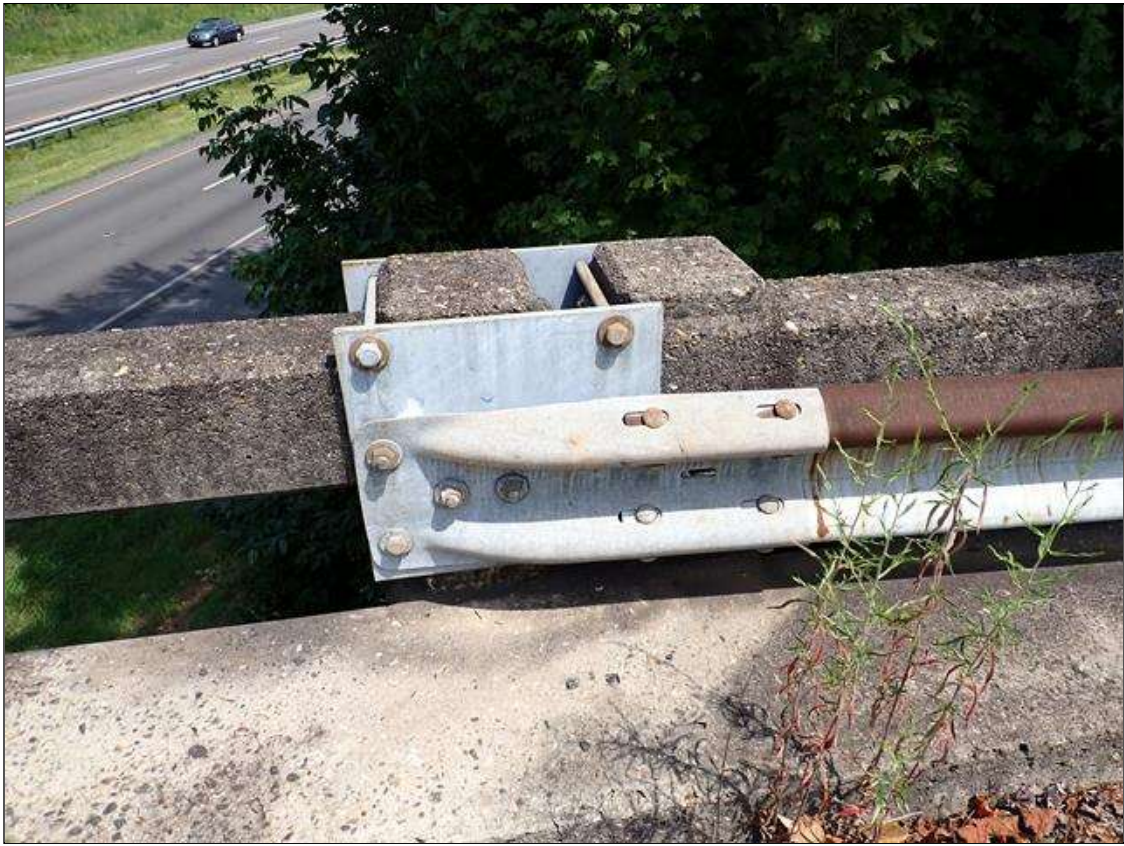
(PAR) southeast guardrail attachment, improper lap
