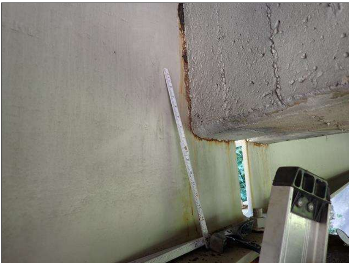
Span 2 Beam 4: at bent 1, web adjacent to end diaphragm, rust scale (10 inch x 15 inch)
