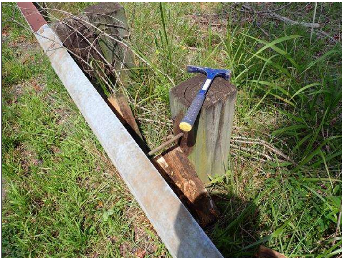
(PAR) northeast guardrail, 3rd and 7th timber posts from end bent 2, timber spacers, missing
