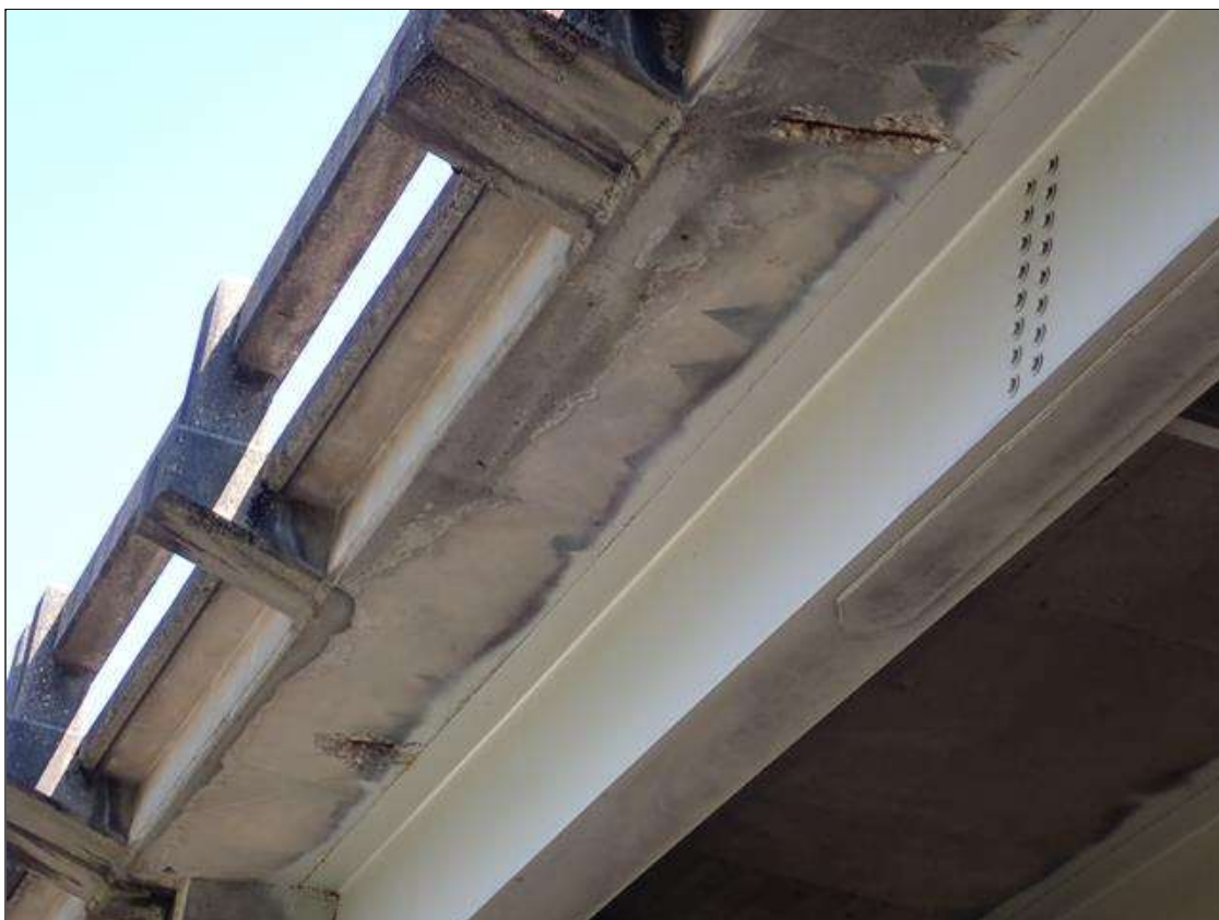
Span 2 Deck: (PAR) along underside of left overhang, two [2] spalls [up to 18 inch x 12 inch x 1 inch deep] with exposed rusted reinforcing [no loss]
