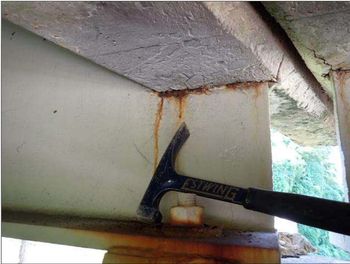
Span 1 Beam 1: at bent 1, corrosion with section loss: web adjacent to end diaphragm (1/2 inch average remaining x 10 inch x 4 inch)
