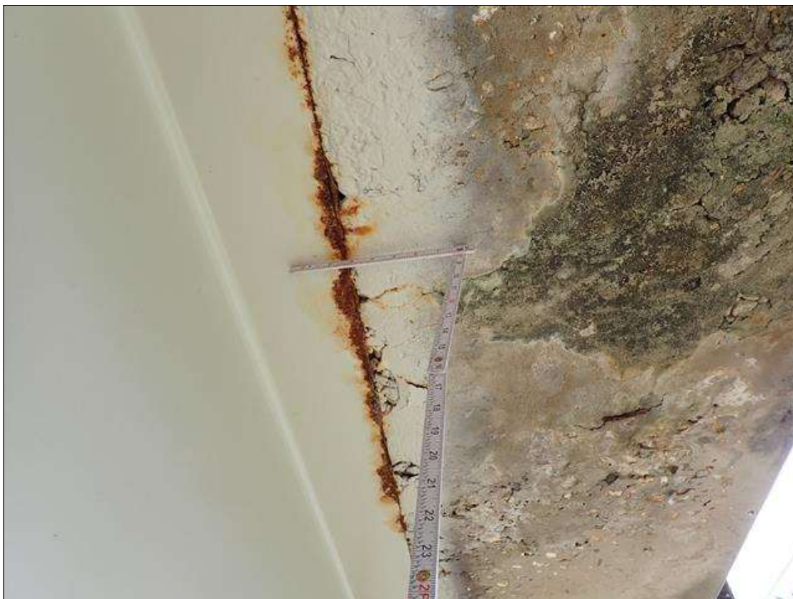
Span 4 Beam 1: West top flange at midspan, active surface corrosion [no loss]
