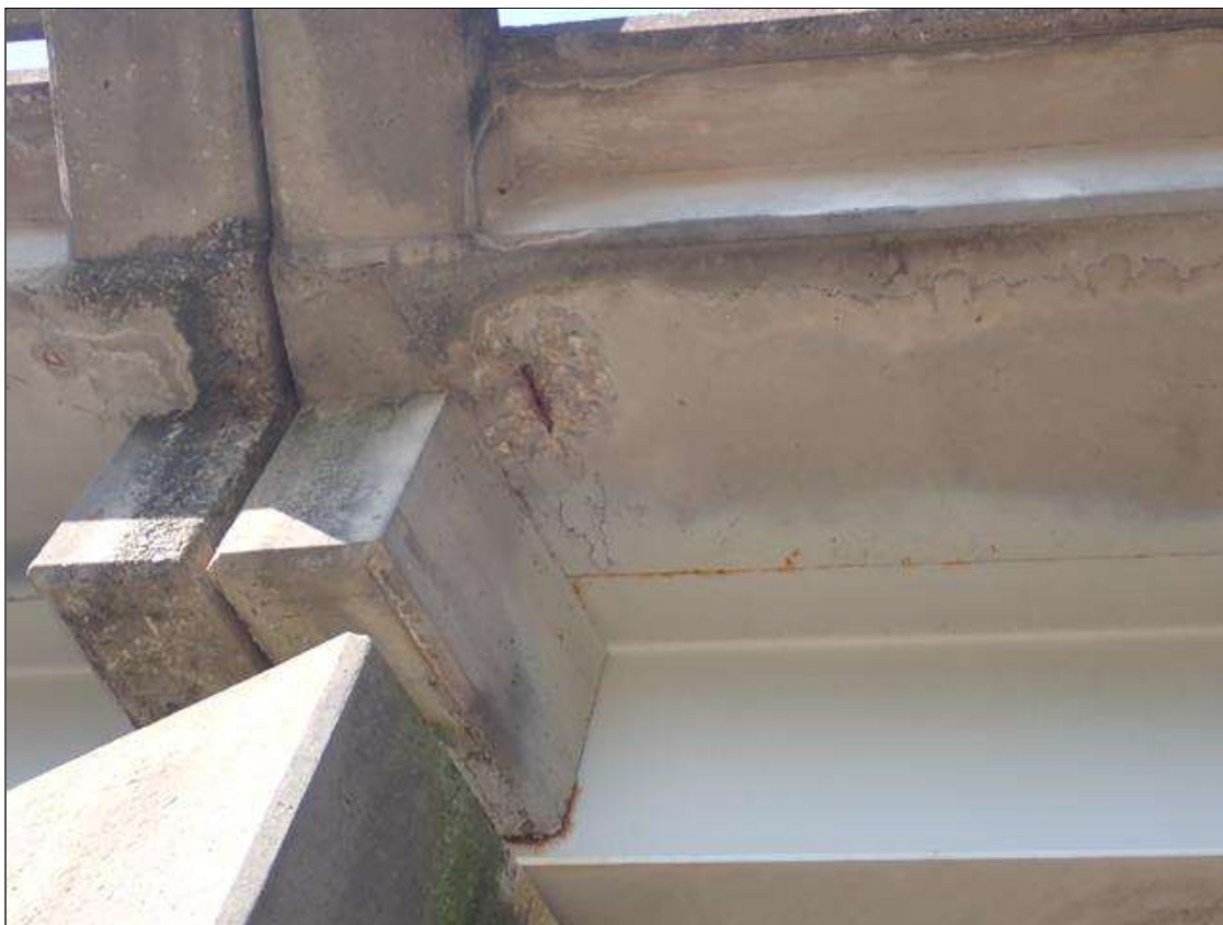
Span 3 Deck: (PAR) MULTIPLE UP TO 1 FOOT X 1 FOOT X 1 INCH DEEP SPALLS/DELAMINATIONS WITH EXPOSED REBAR AT RANDOM THROUGHOUT EAST OVERHANG; SOME DELAMINATIONS OVER TRAVEL LANE
