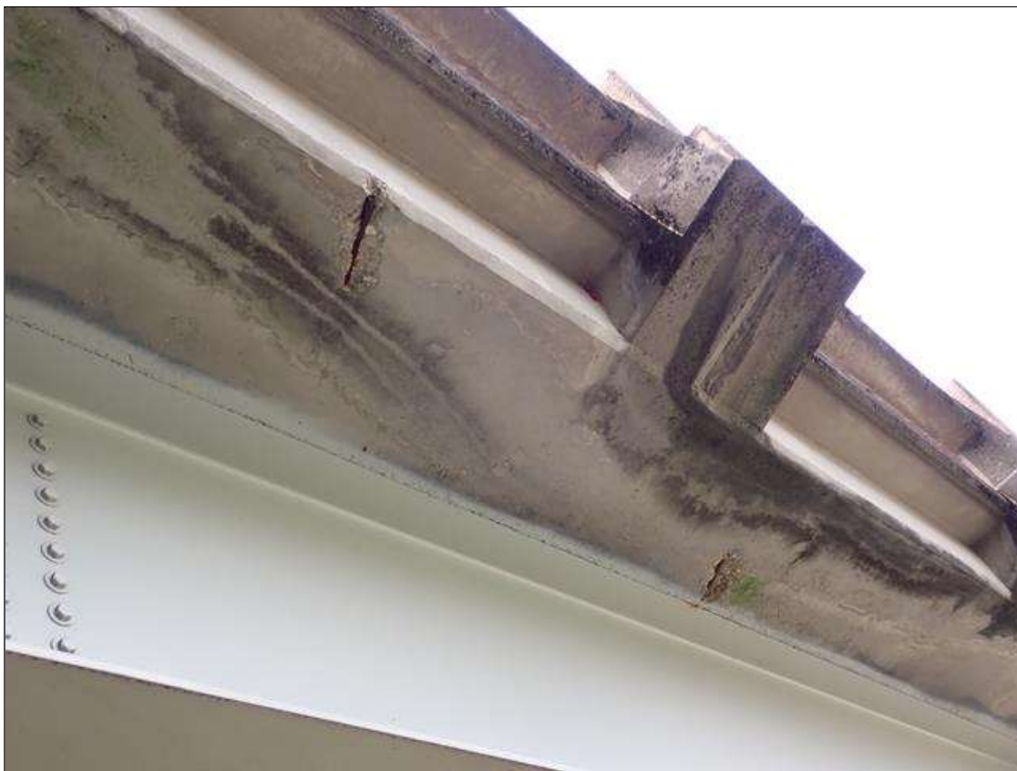
Span 1 Deck: (PAR) [2] UP TO 1 FOOT X UP TO 4 INCH X 1 INCH DEEP SPALLS WITH EXPOSED REINFORCING EAST OVERHANG NEAR MIDSPAN
