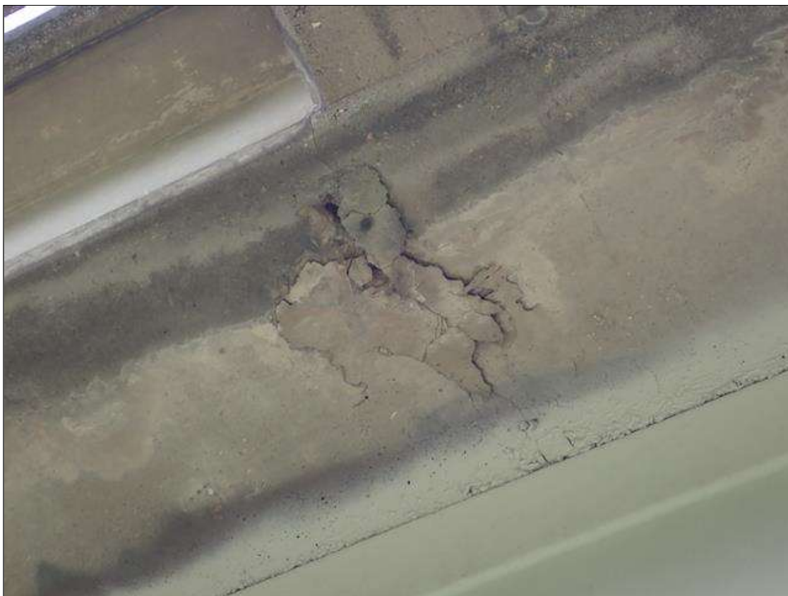
Span 1 Deck: (PAR) 1 FOOT X UP TO 1 FOOT X 1 INCH DEEP SPALL/DELAMINATION WITH EXPOSED REINFORCING WEST OVERHANG 15 FOOT FROM BENT 1
