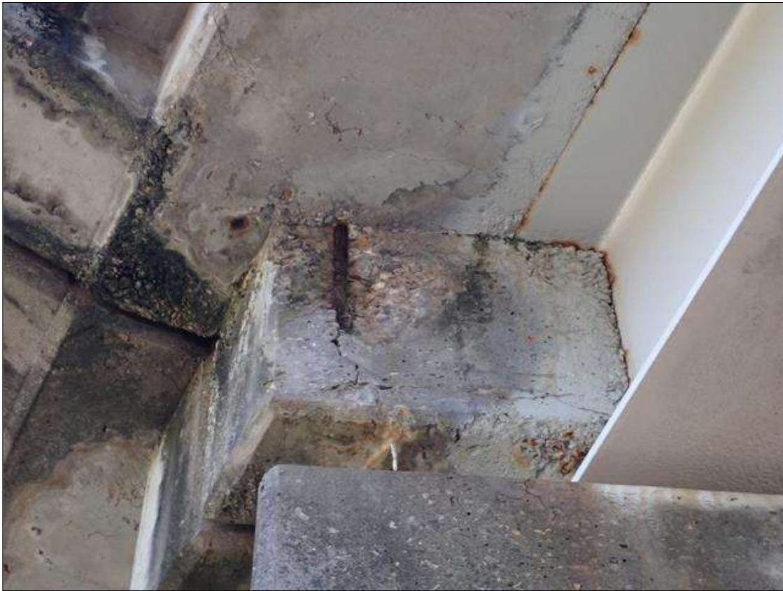
Span 3 Beam 1: (PAR) at bent 3 left overhang end diaphragm, spall/delamination [full height x up to 12 inch x up to 1.5 inch deep] with exposed rusted reinforcing [up to 1/8 inch section loss]
