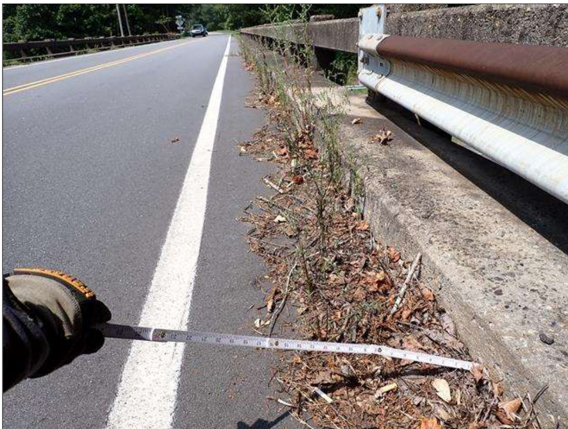
along curblines, debris accumulation (full length x up to 1 foot) with vegetation growth
