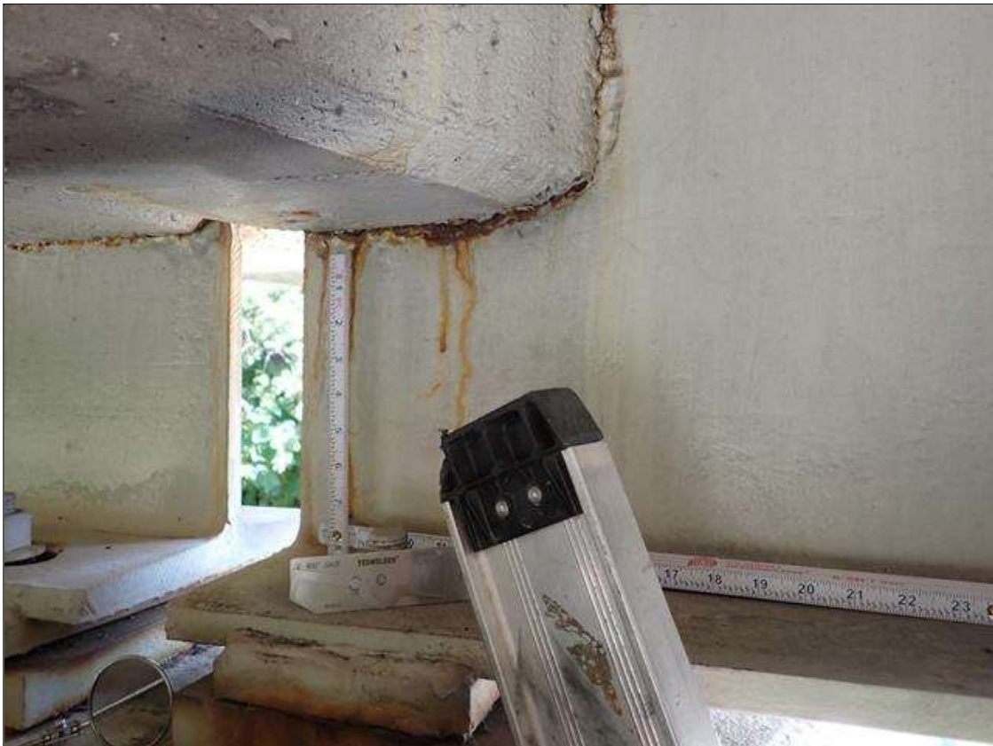
Span 3 Beam 4: at bent 3, corrosion with section loss: web adjacent to end diaphragm (1/2 inch average remaining x 10 inch x 23 inch)
