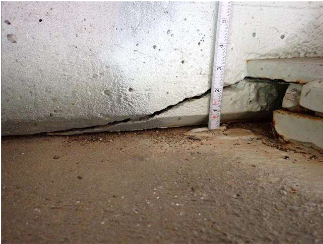
End Bent 1 Abutment: at all beam penetrations, multiple delaminations [up to 9 inch x 2 inch] with cracks (up to 1/4 inch)
