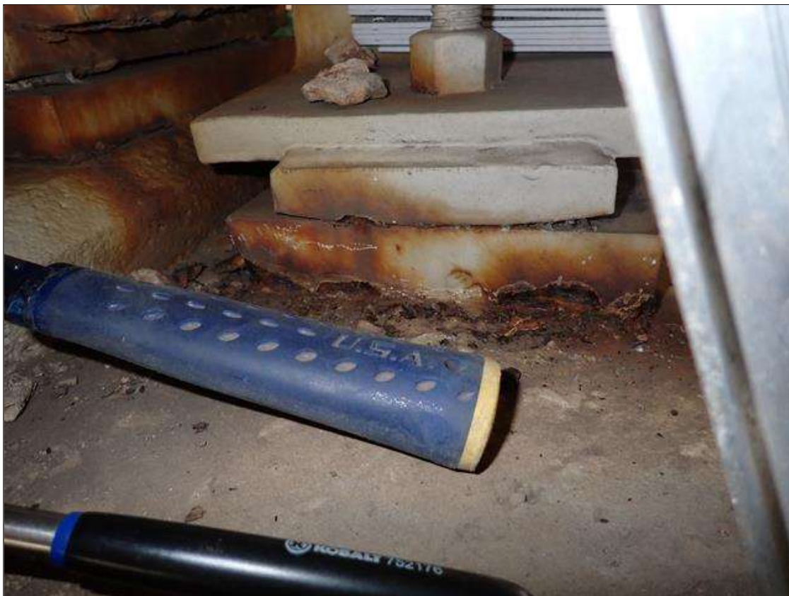
Span 3 Beam 2 - Far Bearing 2: surface rust/rust scale
